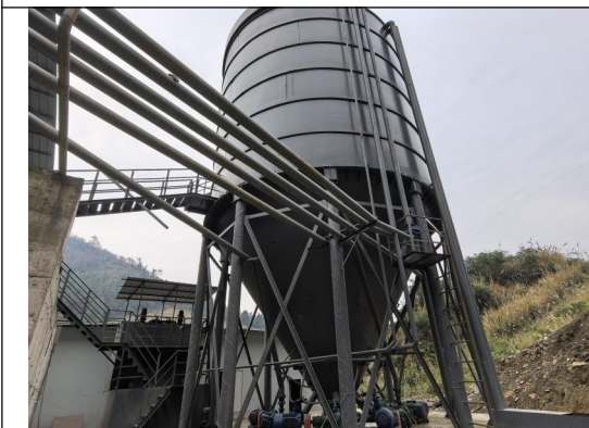
废水絮凝沉淀罐
